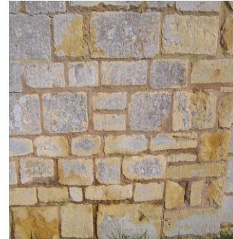
Poorly maintained walls
